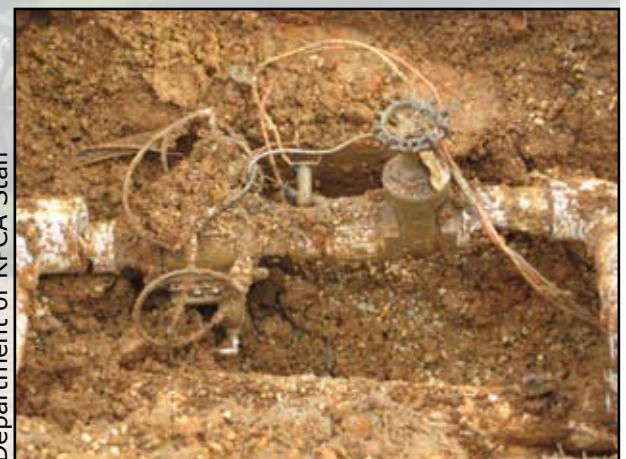
Irrigation Damage from Emergency Vehicles
